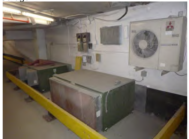
Air Handlers / Air Conditioning Units
