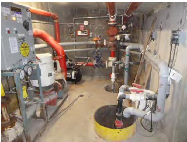
Fire Suppression System / Sump Pumps
