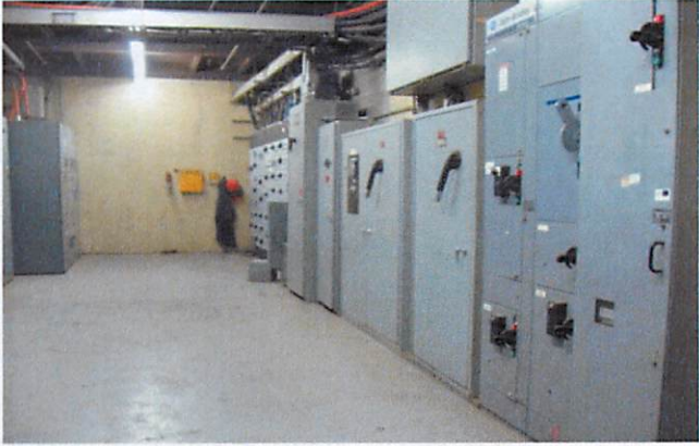
Interior electrical room
